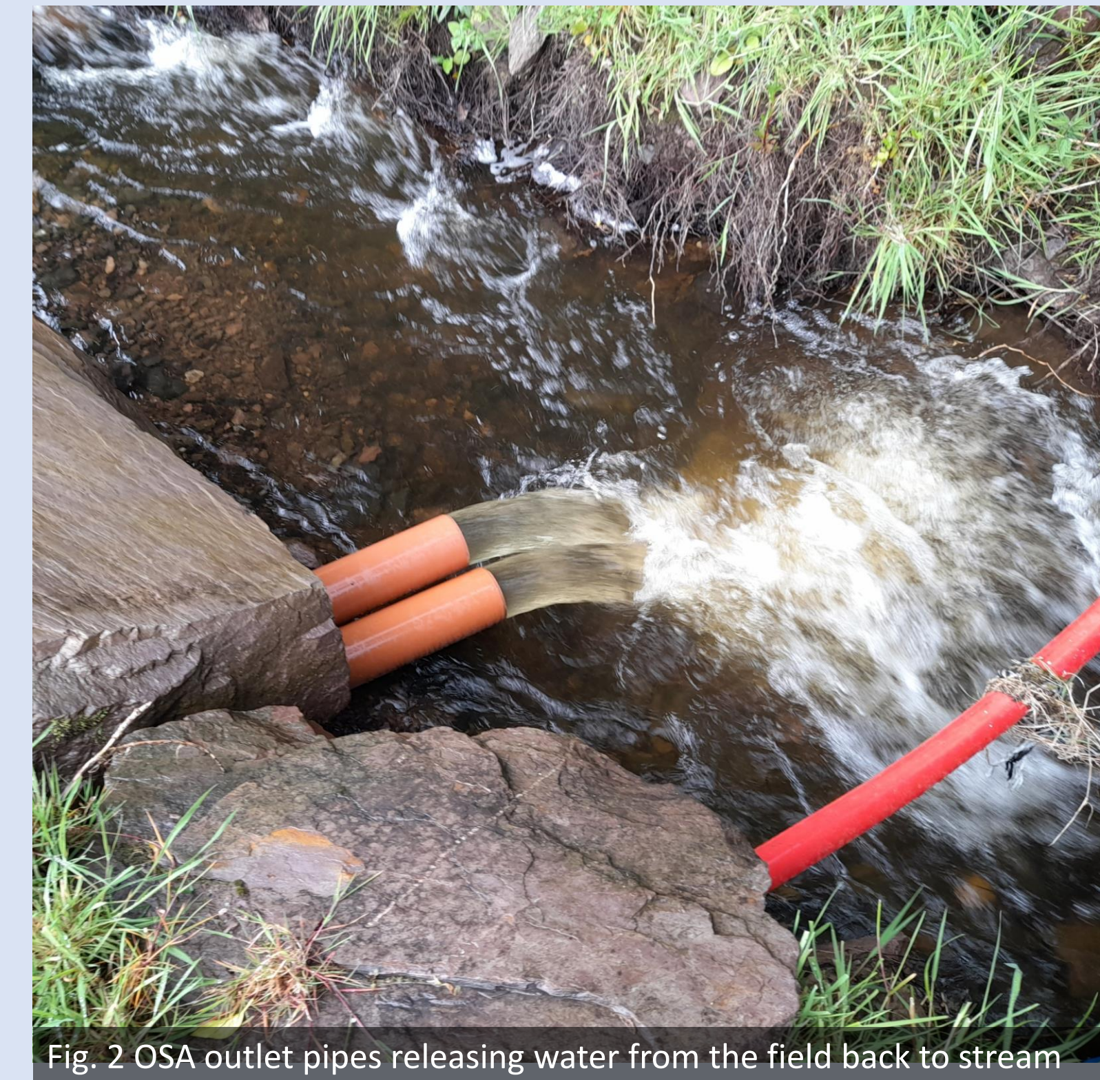
Fig. 2 OSA outlet pipes releasing water from the field back to stream
